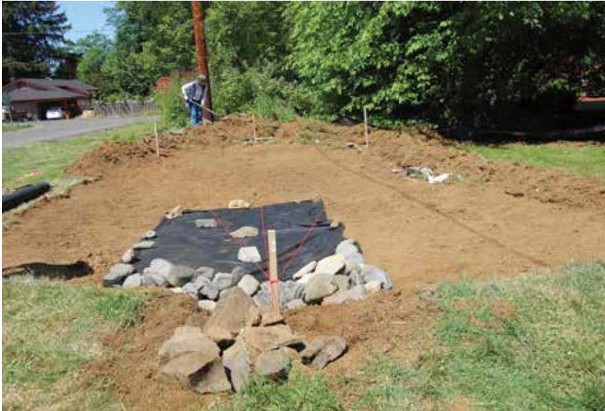
Grading is made simpler by using four stakes, one at the inflow point and three at the opposite or lower end of the rain garden—including, most importantly, the outflow point.
