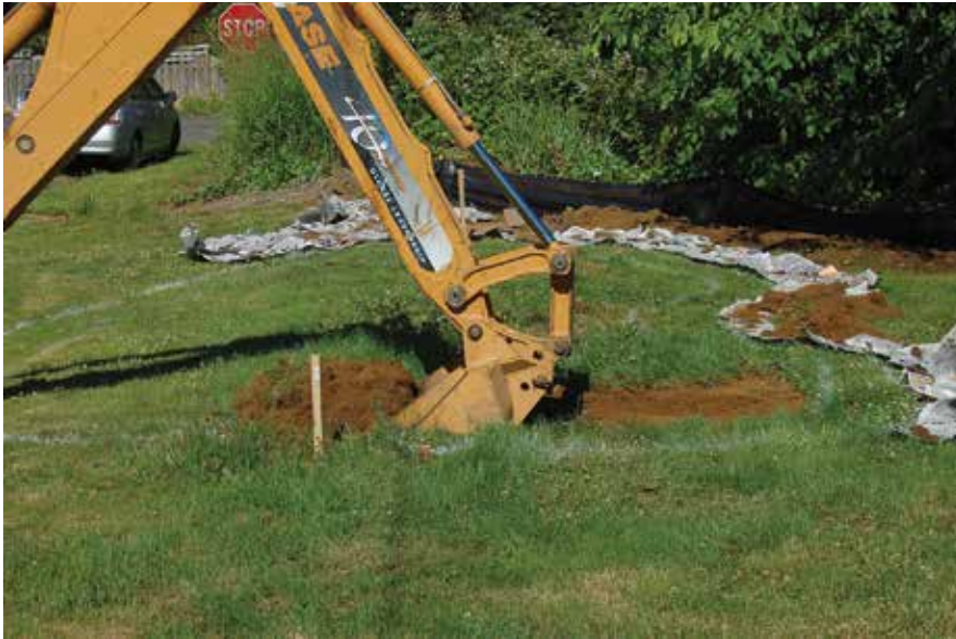
Excavator is located outside of the rain garden in order to make sure the machine does not compact soil in the rain garden.
