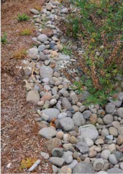
A “dry” stream bed conveys water across a surface before it enters a rain garden.
