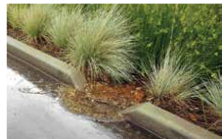
Runoff can enter a facility only if regular maintenance for debris removal is conducted.
